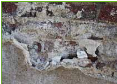
Typical damage through salt efflorescence.
